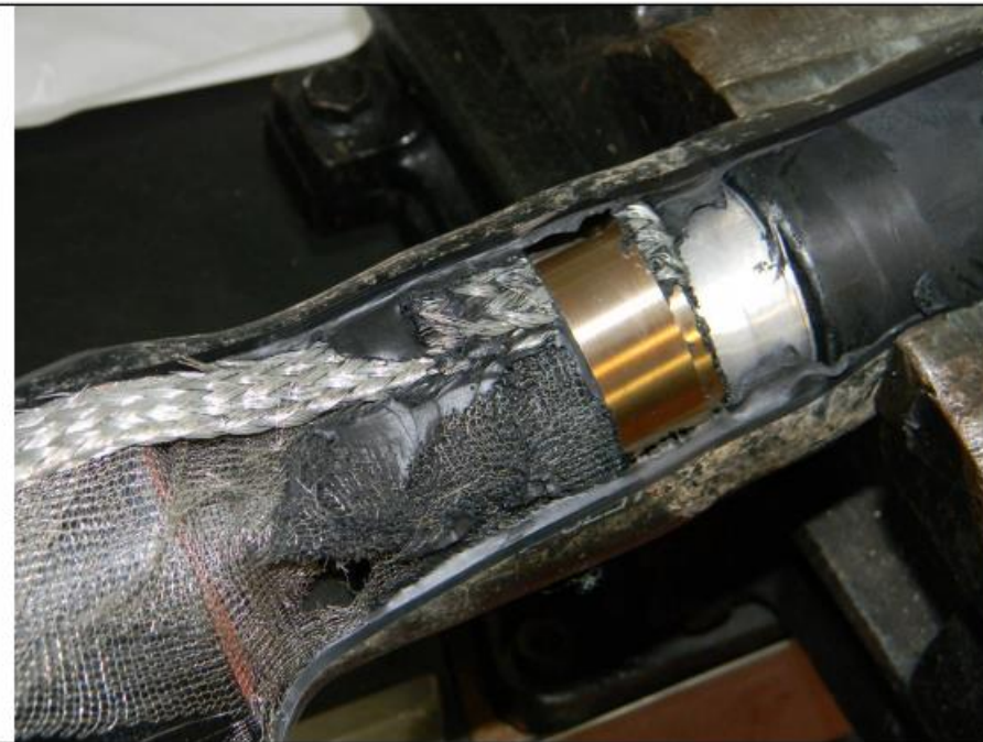
3 - correct contact (joint side B)
