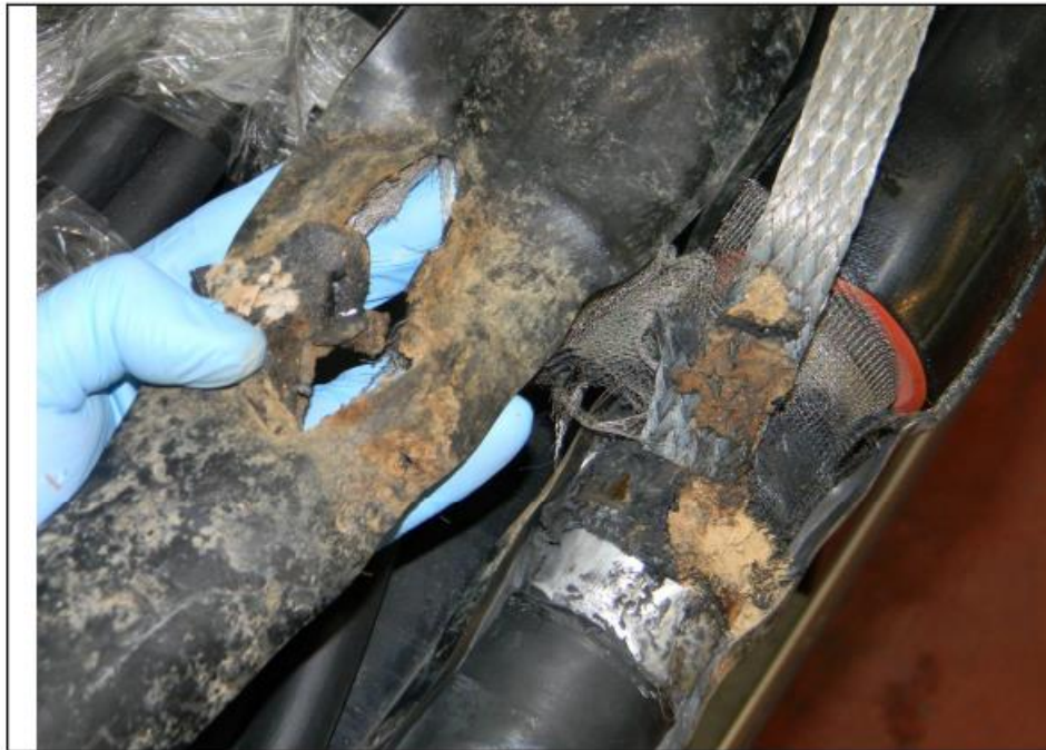
2 - burned contact by high temperature (joint side A)
